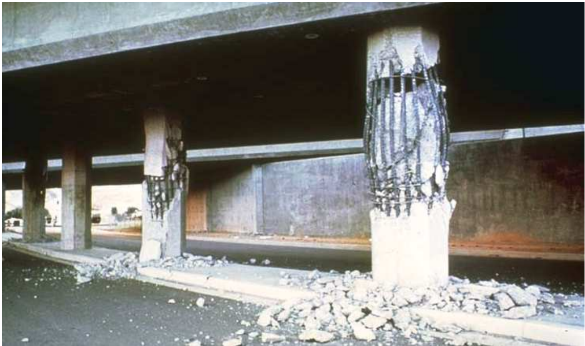
(b) Column damage, Foothills Freeway overpass (USGS, 1971)
