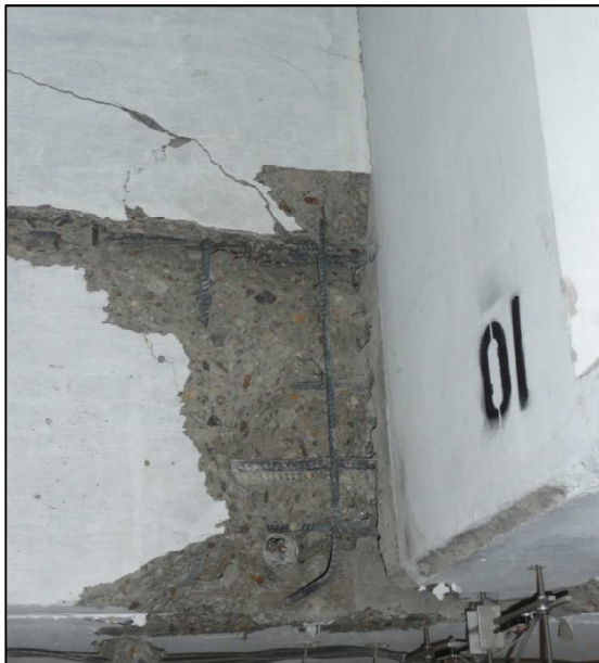
b. Deterioration of as-built connection
