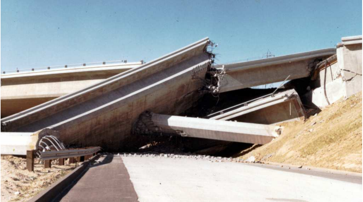
(a) Collapsed highway overpasses, Interstate 5 and Interstate 14 (USGS, 1971)
