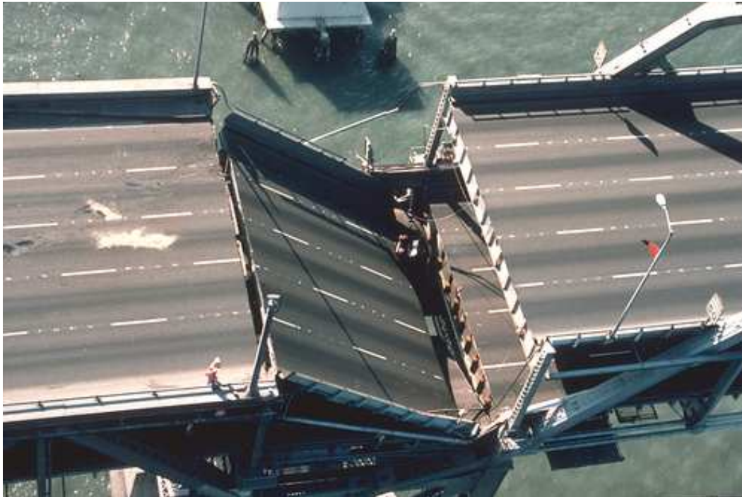
Figure 1.3. Bay Bridge collapse, 1989 (Eskenazi, 2009)
